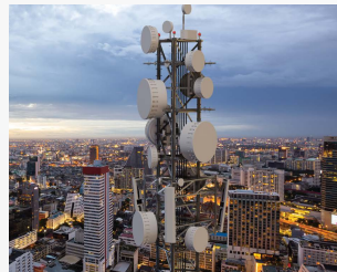
Telecom and Optical Fibre Network
